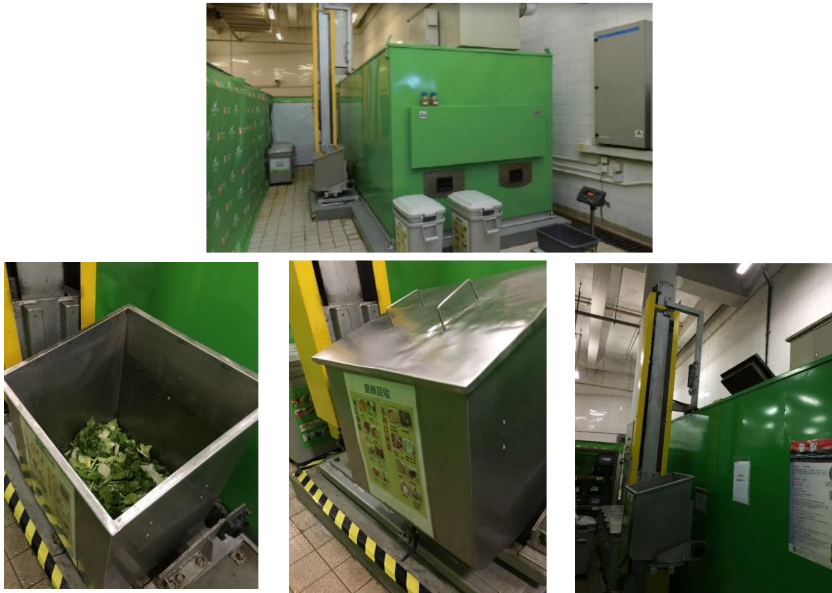
Figure 1: The Highly Efficient Food-waste Decomposer at Olympian City 2
