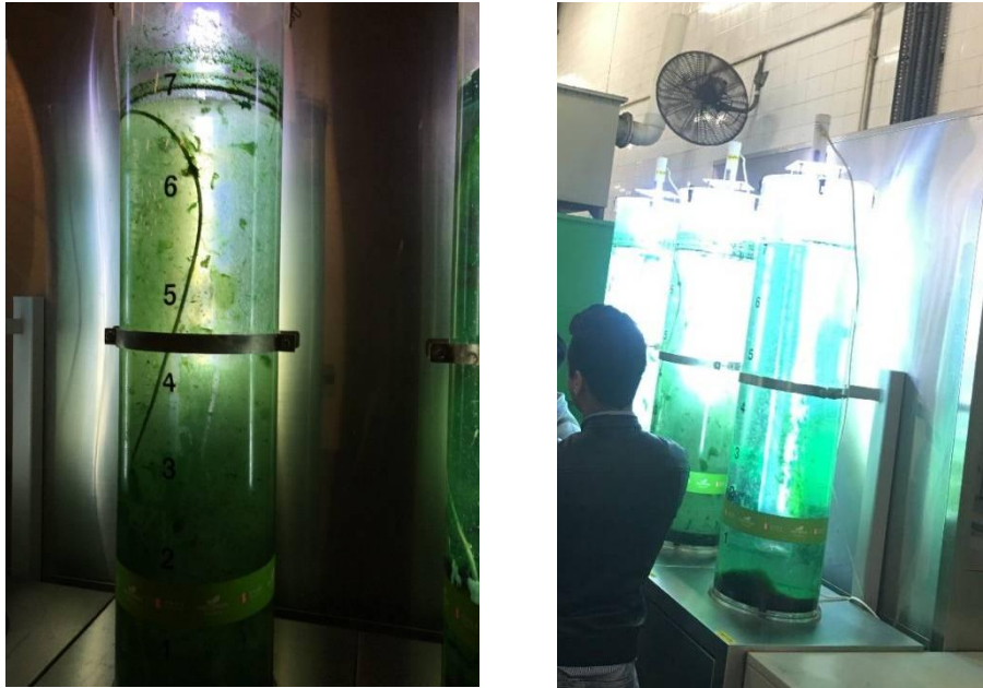
Figure 6: The Microalgae Treatment Setup at Olympian City 2
